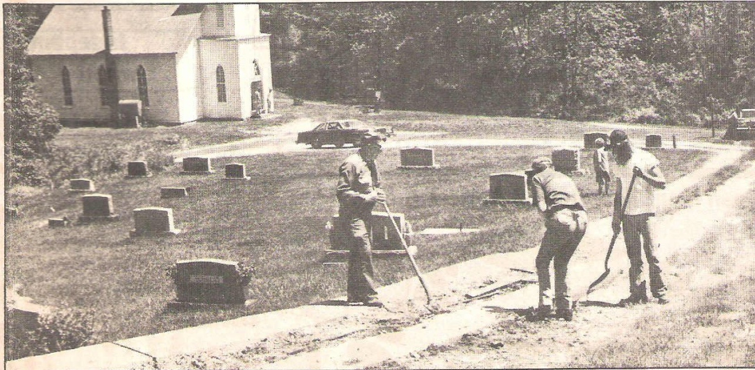
CEMETERY IMPROVED — Bill Hart, Bob Pickett and Robert Pickett Jr., work at the Burlingham Cemetery, finishing the concrete drive in time for Memorial Day.
